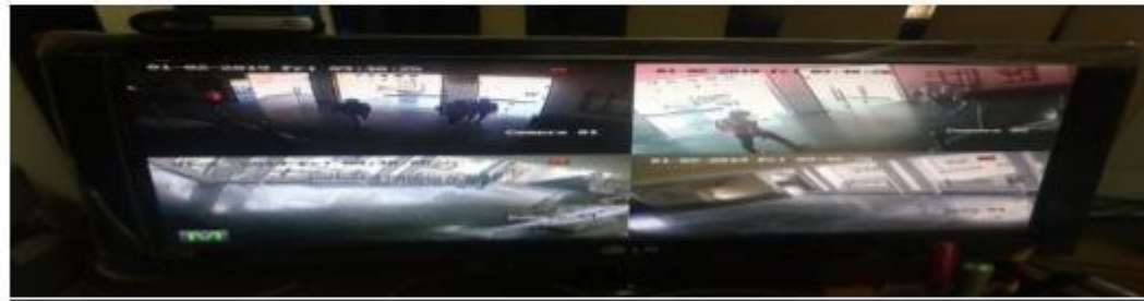
Main entry CCTV Surveillance
