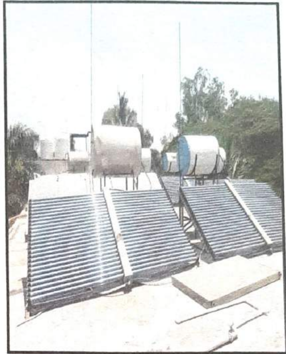
Solar Water Heater
