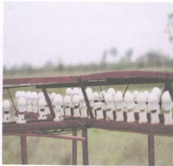
Photo No.3 :Signals system
