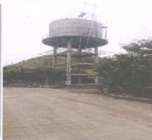
Photo No.2. Water Tank
