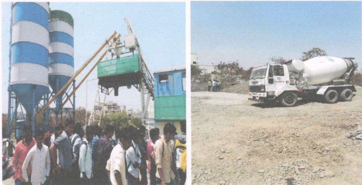
Photo No.2: RMC plant
