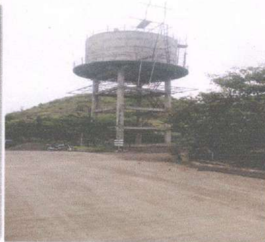
Photo No.2. Water Tank
