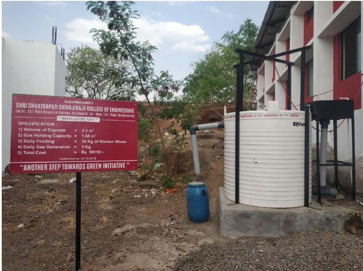
Biogas Plant at Canteen
