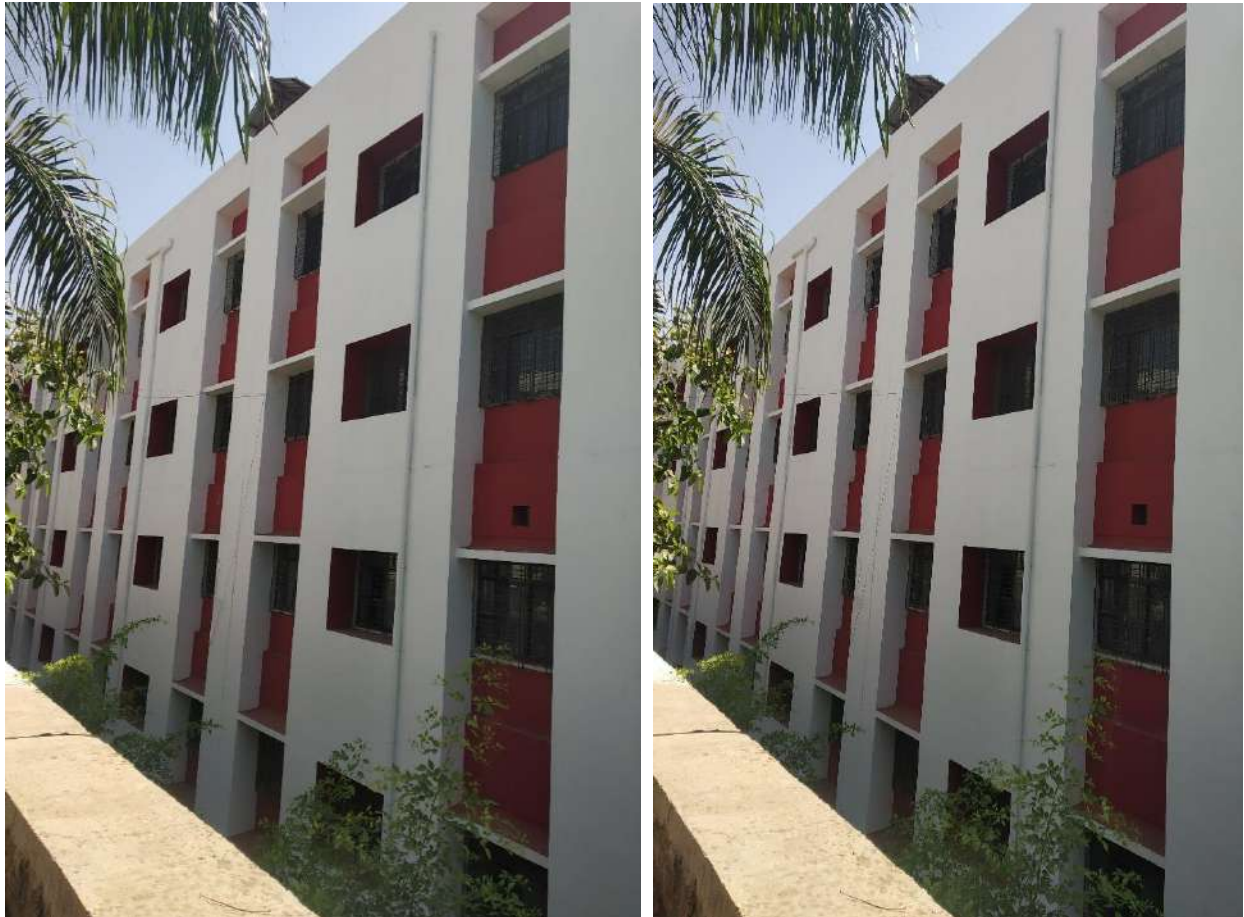
Rain Water Harvesting Pipe
