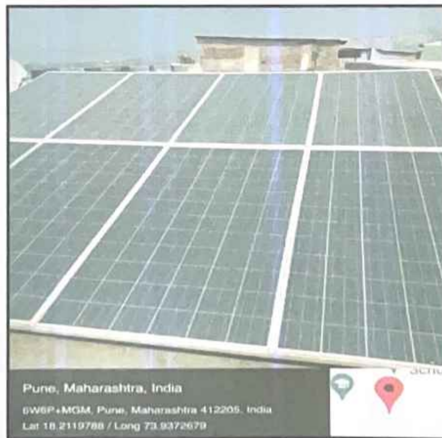
Photograph of 10 kWp Roof top Solar PV Plant:
