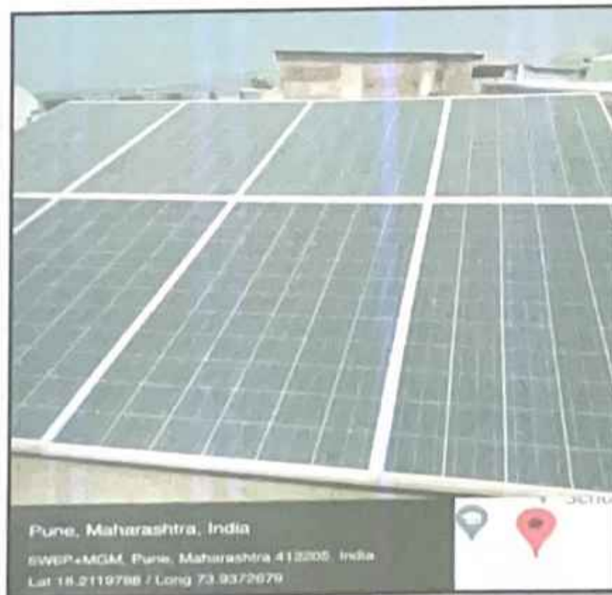
Photograph of 10 kWp Roof top Solar PV Plant:
