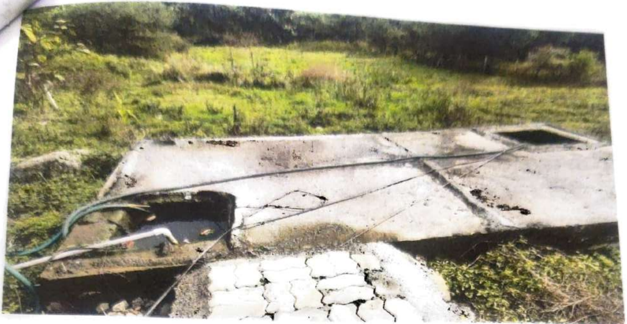
Fig.2: Water intake in kenjal plant
