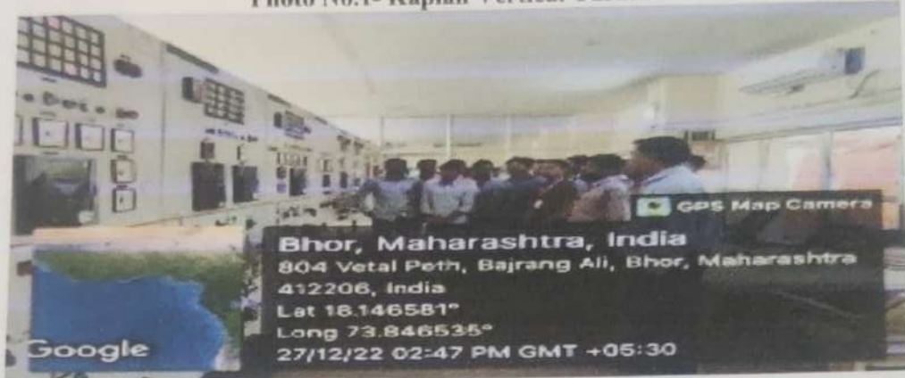
Photo No.-2 Control Panel system
