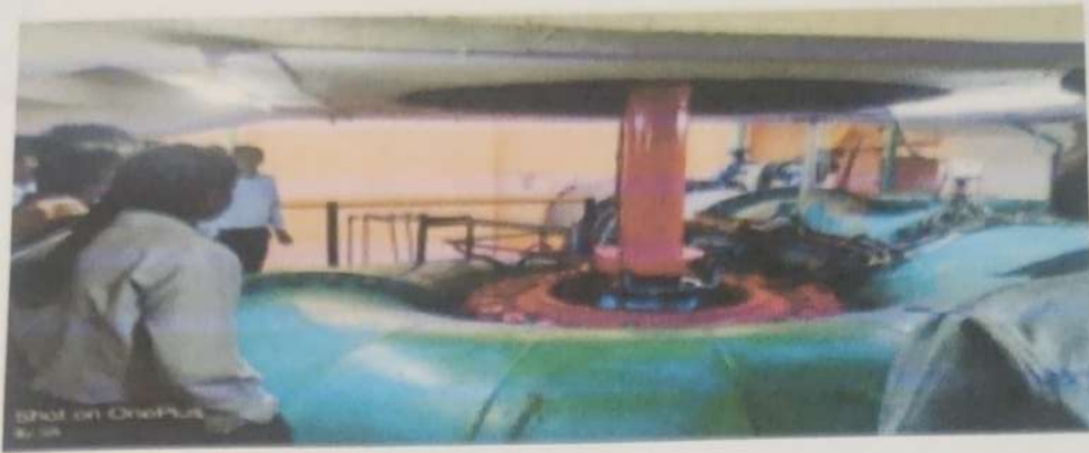
Photo No.1- Kaplan Vertical Turbine
