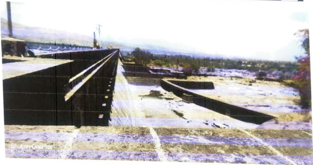
Photo.No.2-Stilling basin & Automatic Gate
