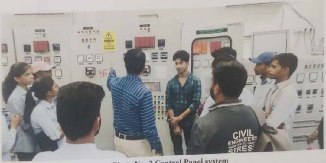
Photo No.-2 Control Panel system
