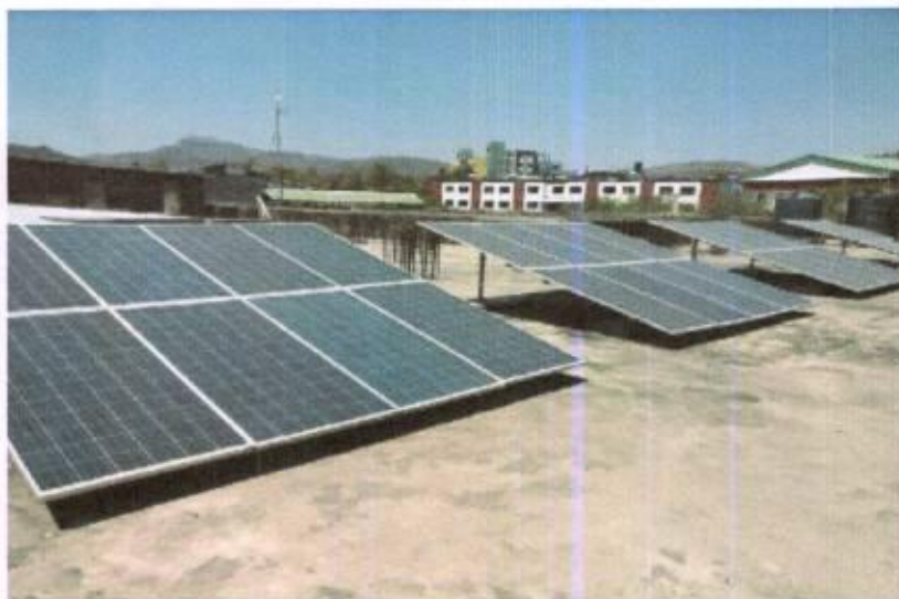
Photograph of 10 kWp Roof top Solar PV Plant:
